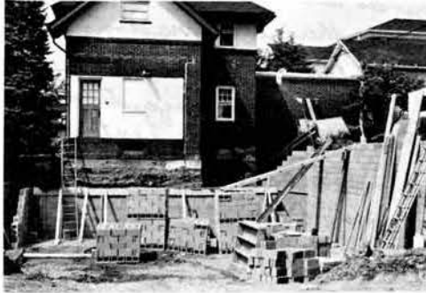
The above shot shows construction progress as of Aug. 10. Photo by S. Pennington
