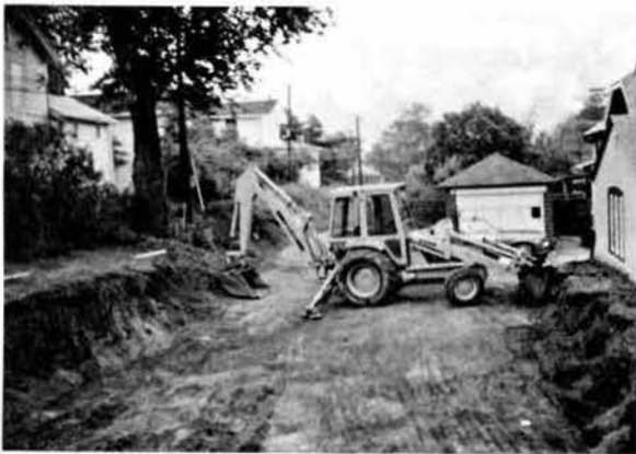
South view of the backyard--Garage is gone. Excavation is well under way. Photo by S. Pennington
